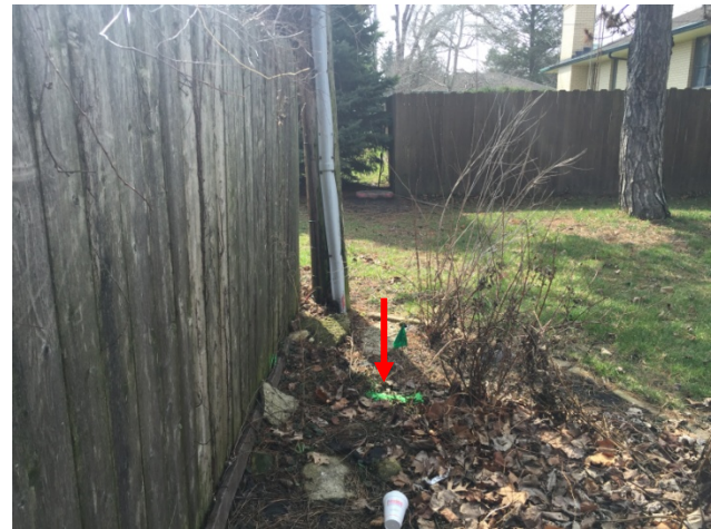
#4: Approximate Point Repair (PR) Location Looking SW (810 Grand's Backyard)
