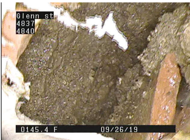
#5: Collapsed Lateral from Mainline
