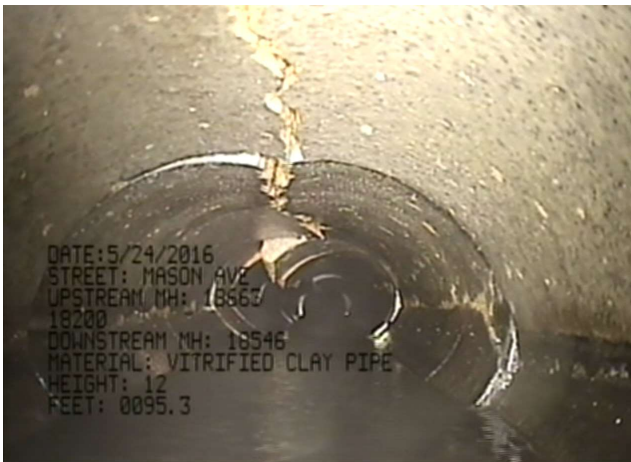
#5: Deformed Pipe from Upstream
