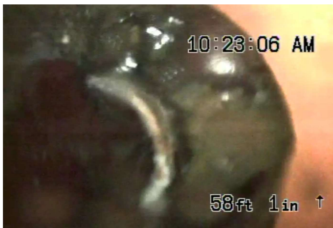
#5: Collapsed Service from Lateral
