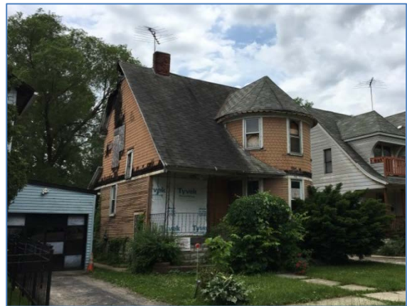
FIGURE 2: FIRE DAMAGE AT 220 LINCOLN STREET
